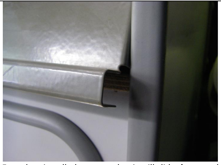
Faceplate is pulled away so that it will slide down and clear the plywood
